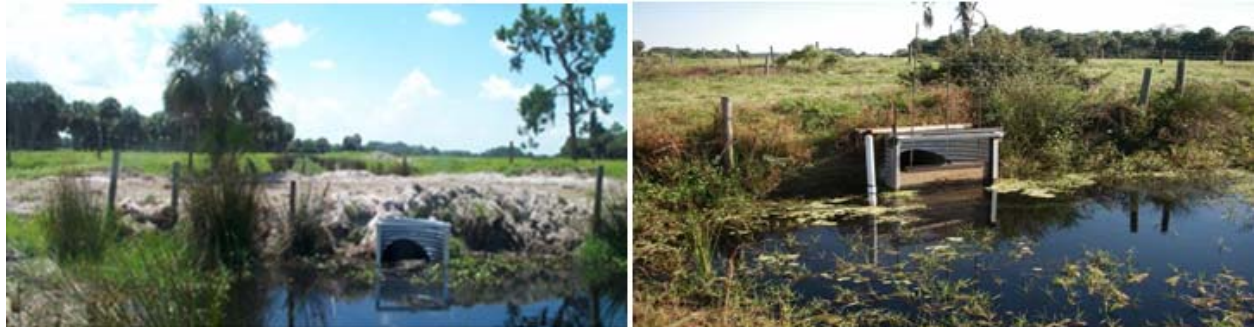
Figure B-7. Wetland 1 outlet with only the culvert during the pre-hydration period (left) and with the culvert and flashboard riser during the post-hydration period (right).
